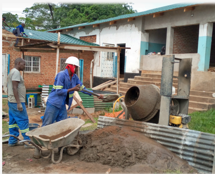
New Postgraduate Studies Centre currently being built photos kindly shared by Ken Ross
